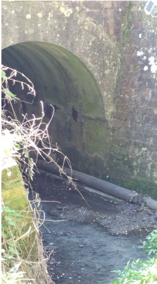
18. Flow in culvert from Black Bears Polo club. Origin of flows although there is a small pond on the west side of the railway line.
