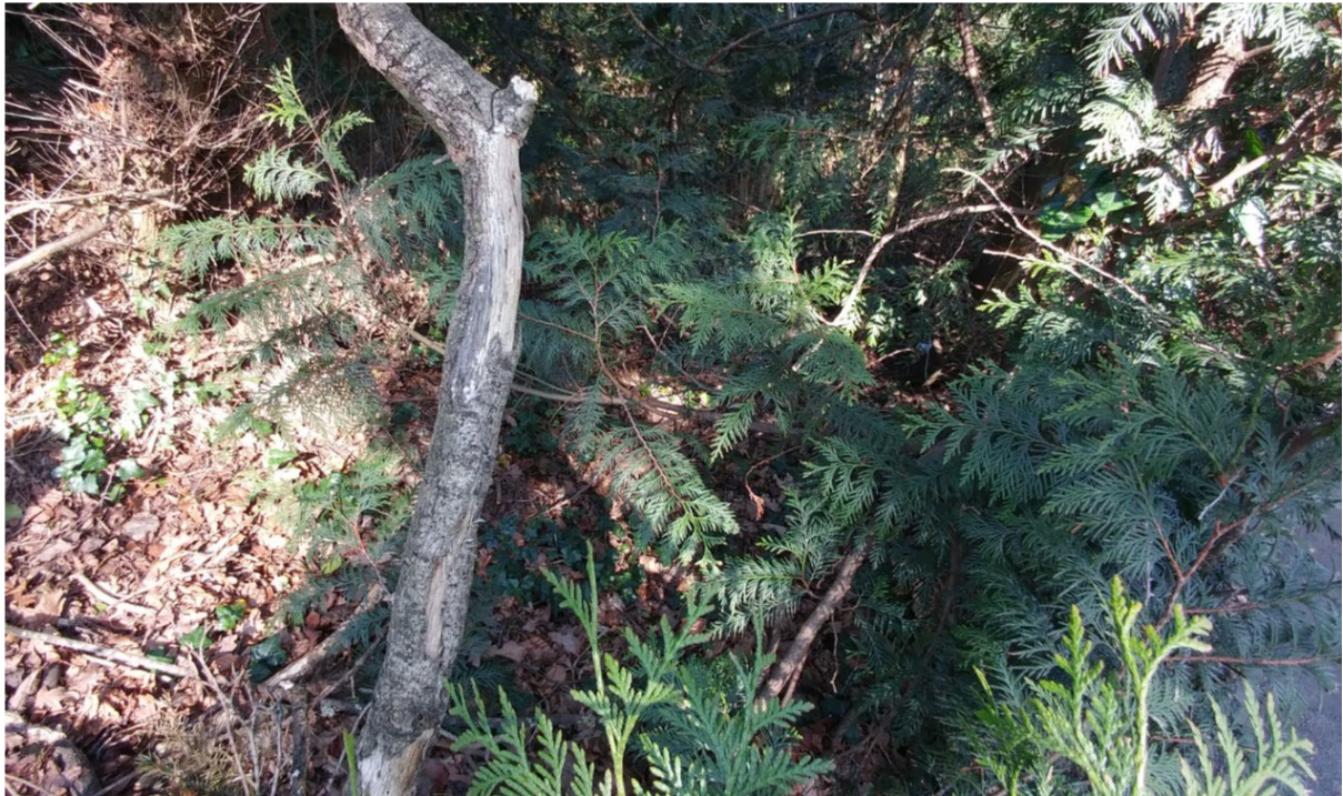
38. Deep ditch on opposite side of road beside private road probably serving existing few gullies locally. Possible drained to existing highway drainage to the east.
