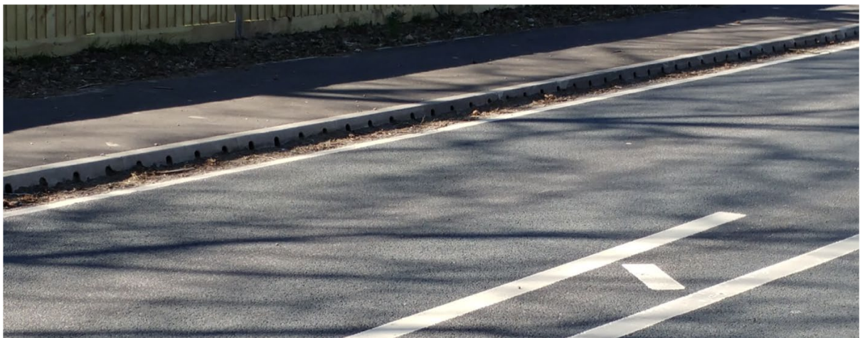
37. Beany blocks drainage of A4155 (all along the road beside development site)
