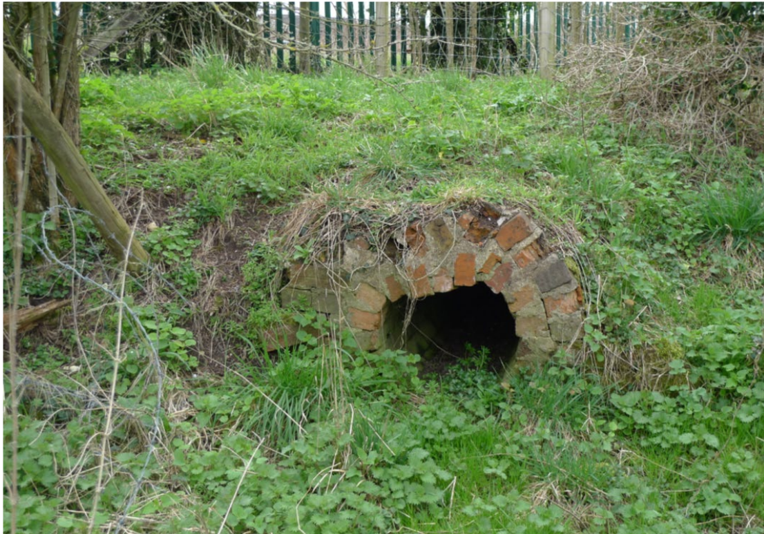
9. Very old 450mm culvert serving AFC ditch passing flows from ditch to railway culvert.
