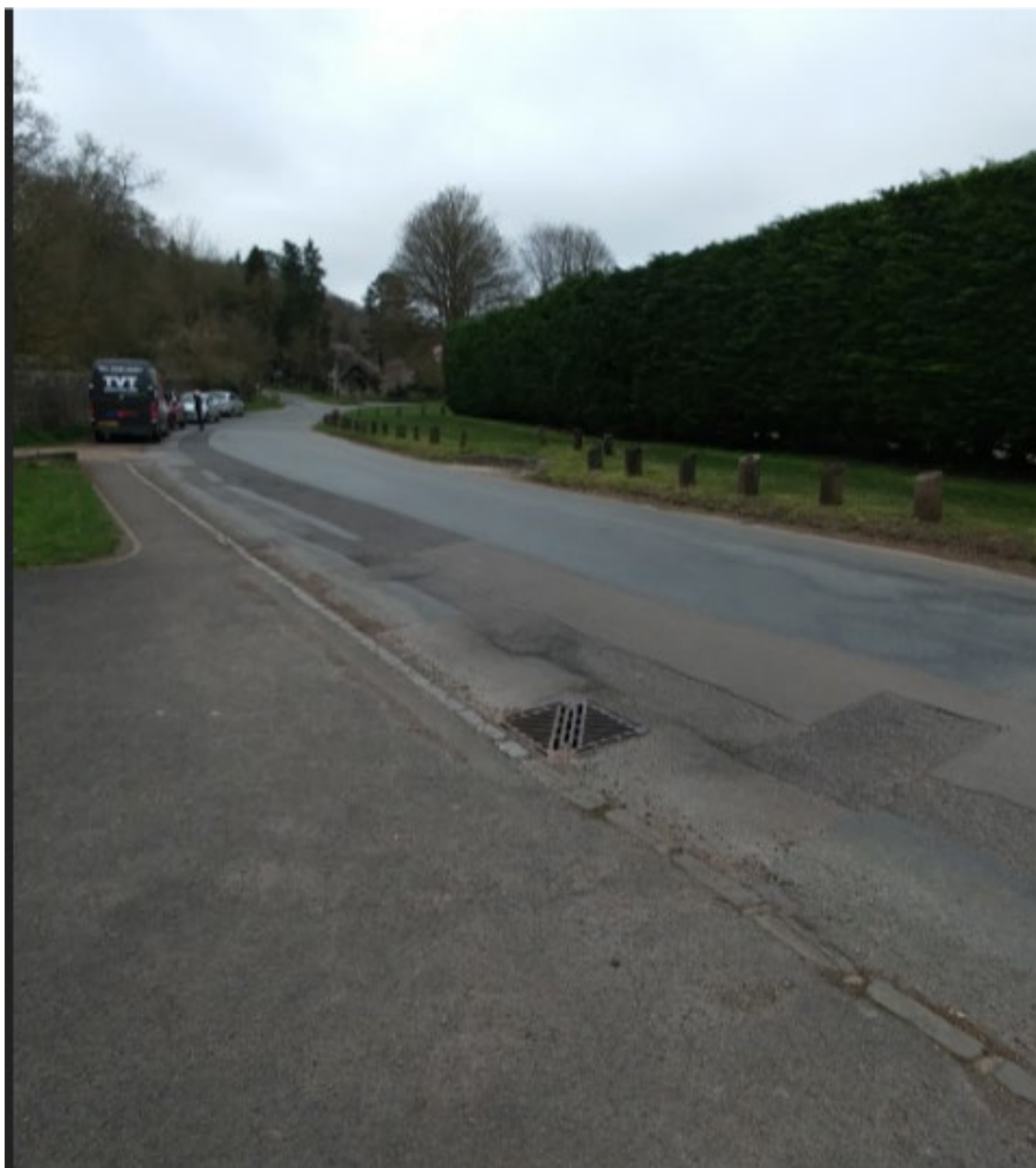
34. Uphill from church looking up road to Sonning Common. Gullies connected to inflow to pond (to be rectified soon).
