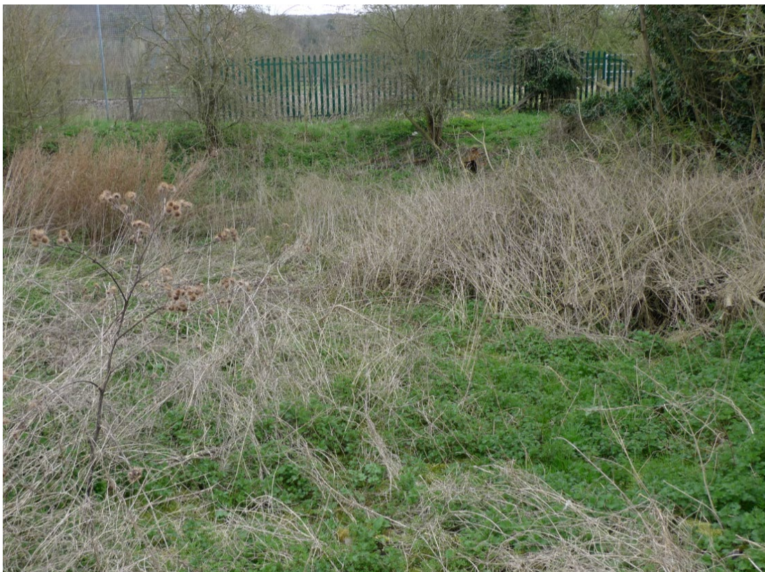
10. Very old 450mm culvert serving AFC ditch and ponding (waste) area.
