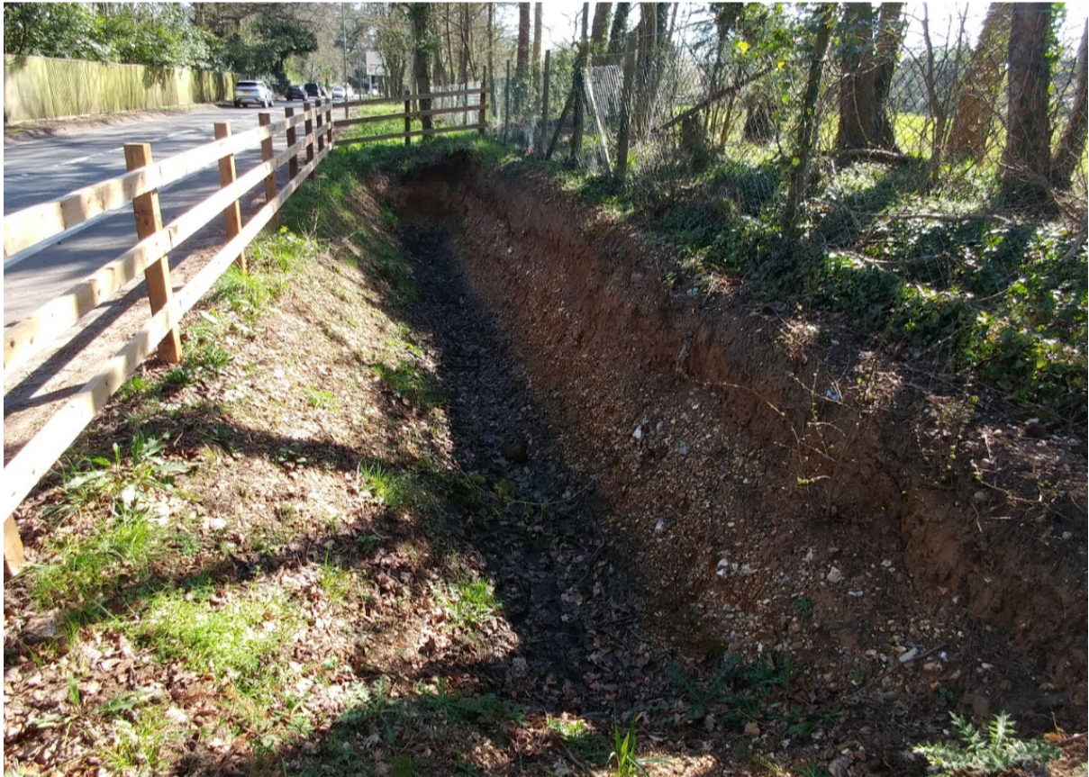
36. Deep ditch cut by developers beside A4155 – no apparent inlets or outlets.
